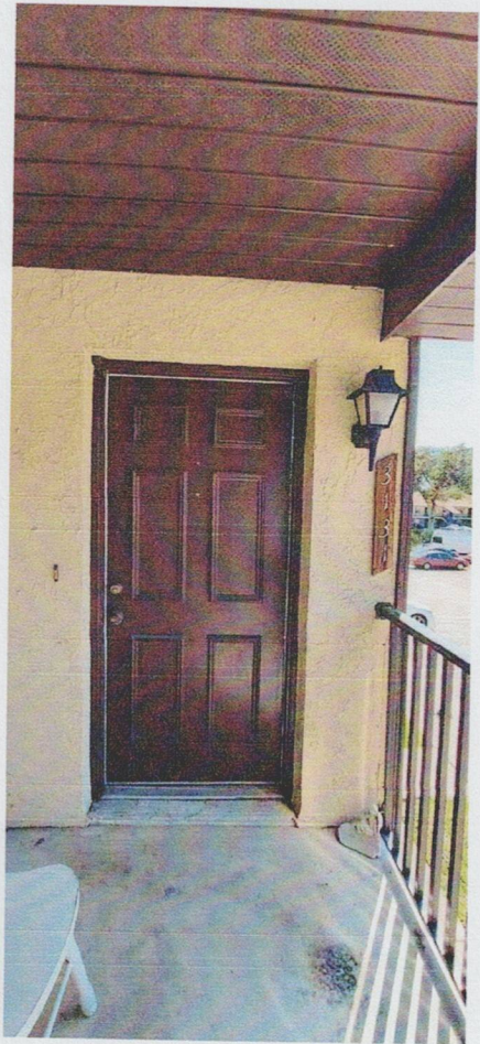
Unprotected non-glazed entry door
