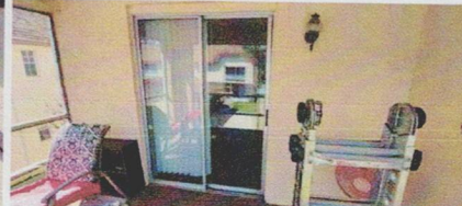
Unprotected glazed entry door
